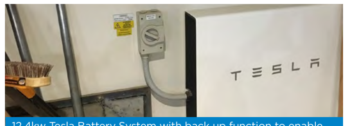
12.4kw Tesla Battery System with back up function to enable use during power outages.
