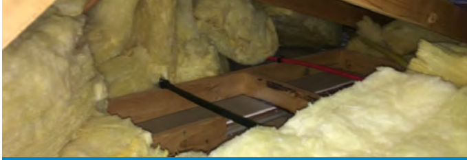
A number of areas were identified that were missing insulation. These will be rectified by the builder.
