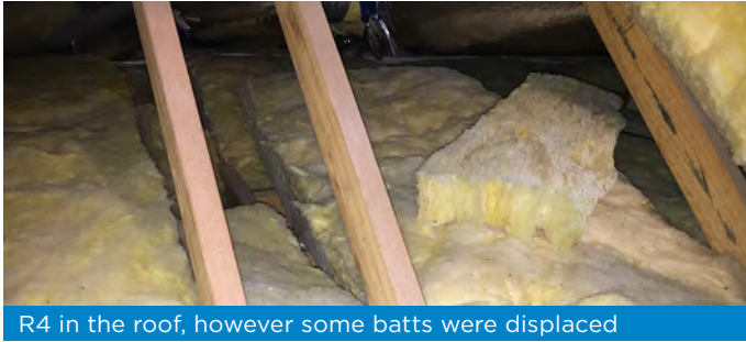
R4 in the roof, however some batts were displaced
