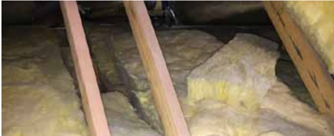
R4 in the roof, however some batts were displaced
